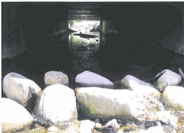
New fish passable concrete box culvert (12' x 6' x 80') under Canterwood Blvd. NW
